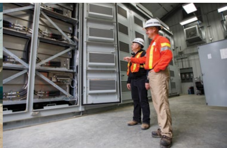
Trevor Wareham, BC Hydro Electrician Sub-foreman, and Vlad Kositsky, BC Hydro Project Manager, inspect one of four banks of sodium-sulphur battery modules. These four banks of battery modules, linked together, create the one megawatt capacity. Photo courtesy of BC Hydro and Power Authority.
