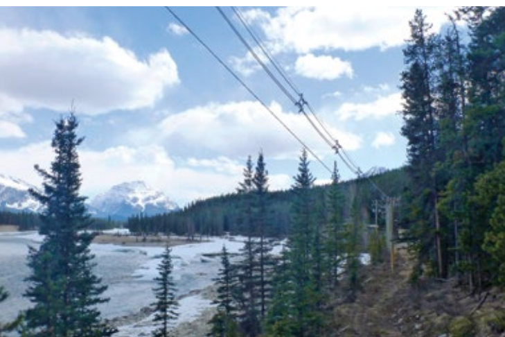
A section of the newly-installed aerial spacer cable system along the Astoria River. Photo courtesy of ATCO Electric.
